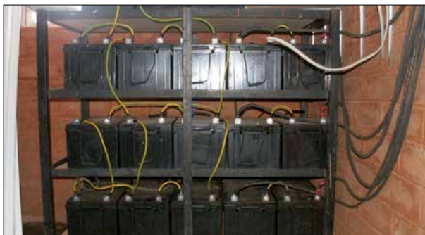
Figure 11: Batteries and battery chargers
