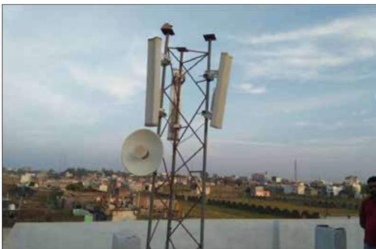
Figure 6 - Tower with three transmitters and one receiver
